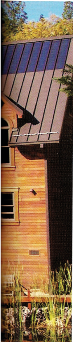
Amorphous-film photovoltaic laminates are adhered directly to standing-seam metal roofs. Photo courtesy of Uni-Solar, Auburn Hills, Mich.
